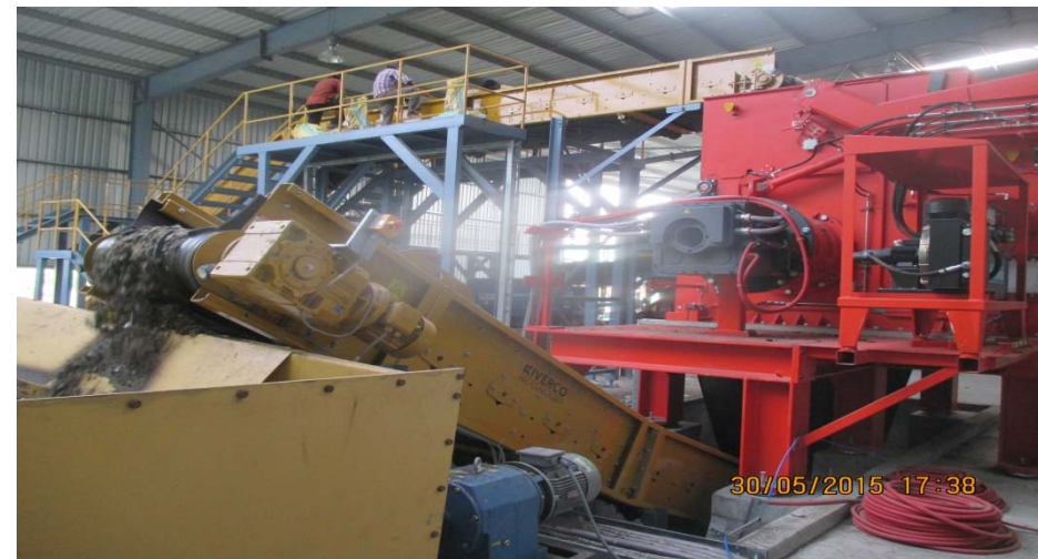
SECONDARY SHREDDER & CONVEYORS
